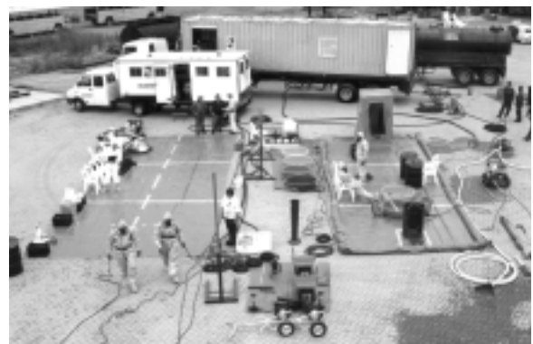
A view of the project’s staff and PPE decontamination system on the right hand side, the PPE donning area on the left and the mobile medical station in the background.
