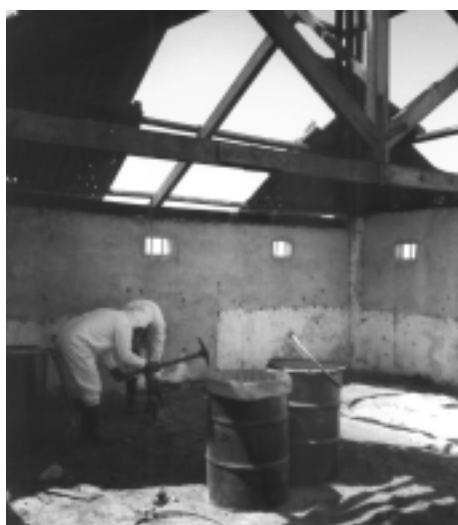
An example of the structural neglect found in some stores. At this store located in Nampula Province crew's were required to excavate compacted product and soil from an unlined floor.
